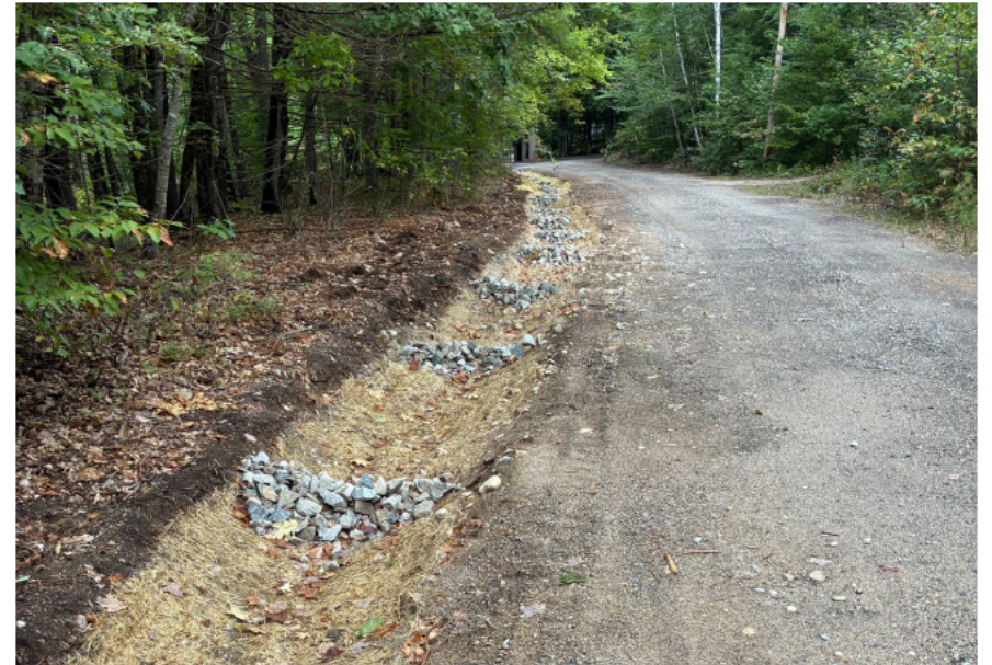
Roadside swale revegetation with rock check dams for sediment and erosion control.
