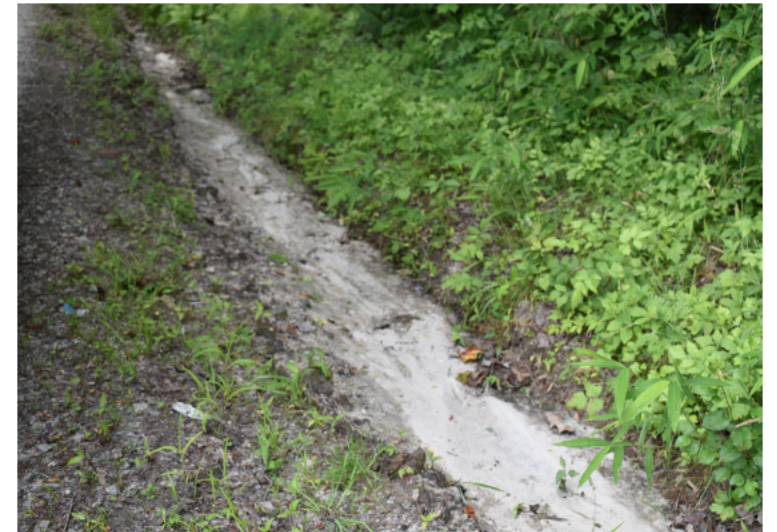
Sediment infilling a roadside ditch in the Upper Chauga watershed. Photo: Steven Pruitt
