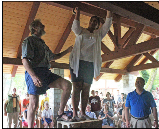
Cissy Henry, Clayton City Manager, drives the last peg into the timber frame pavilion at Stekoa Creek Park.
