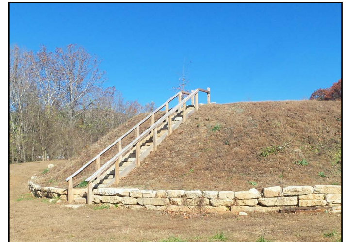
Steps and a retaining wall were constructed from the salvaged concrete, to stabilize a large mound of fill dirt next to Hwy. 441.
