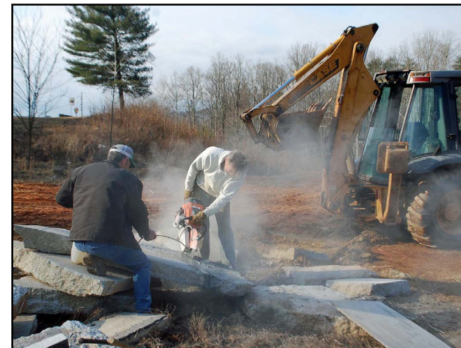
Mounds of concrete dumped on the park site were unearthed and laboriously cut into manageable blocks for building materials.
