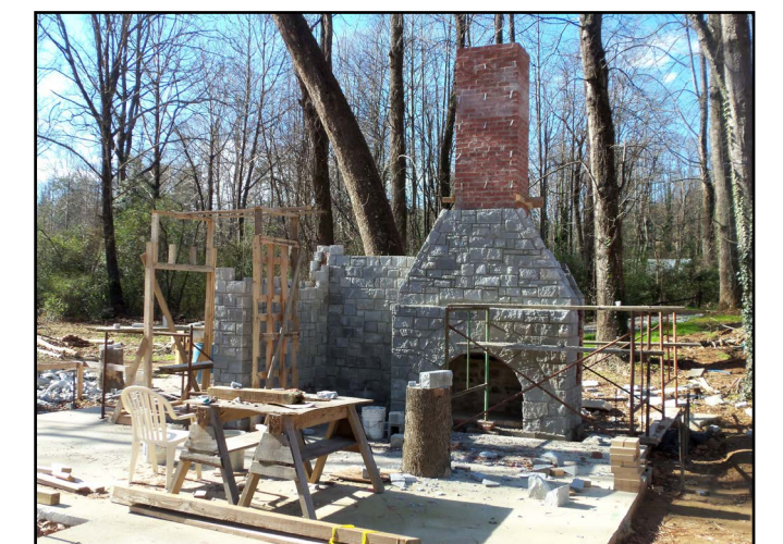
Construction is underway of a community pavilion, that will be a replica of a local structure built by the Civilian Conservation Corps.
